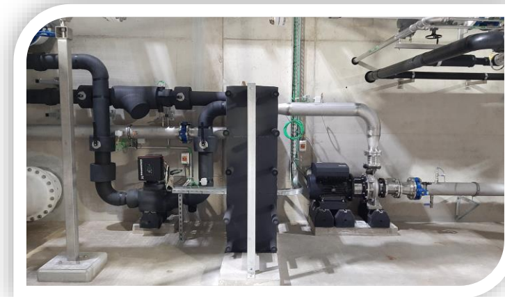
Hydro energy project – heat exanger
